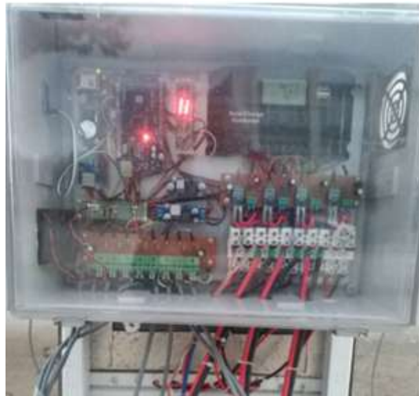
Figure 2. Data logger system used for recording PV panel voltage and current values
